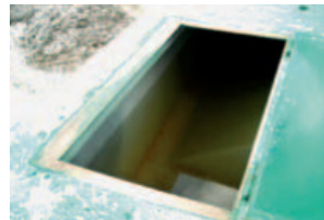
Separate cabinet area stores liquids to be pumped out easily.
